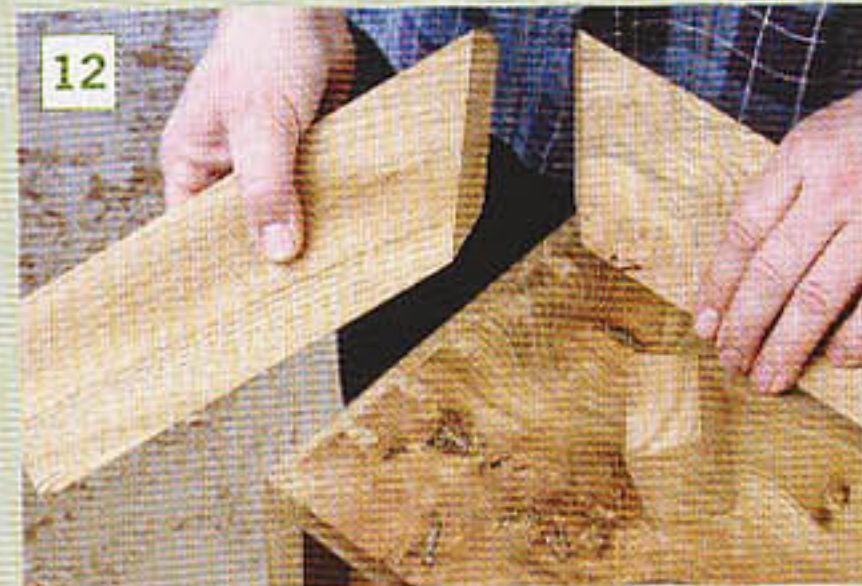
12 The cornice is cut at a compound angle with a block cut to fit inside
