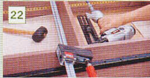
22 The sides are assembled with the top and fixed shelves using glue and 18g brads to keep it all together
