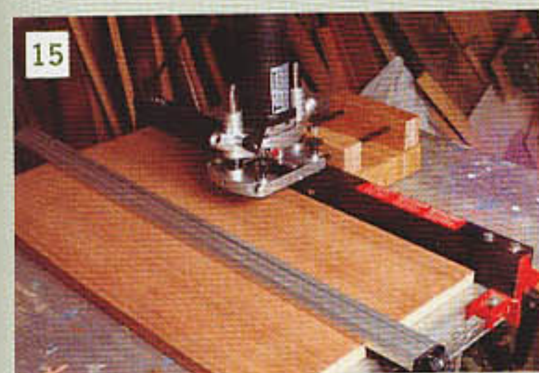
15 The final assembly ready for operation
