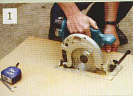
1 The initial breaking down is best carried out with the sheet resting on skids on the floor
