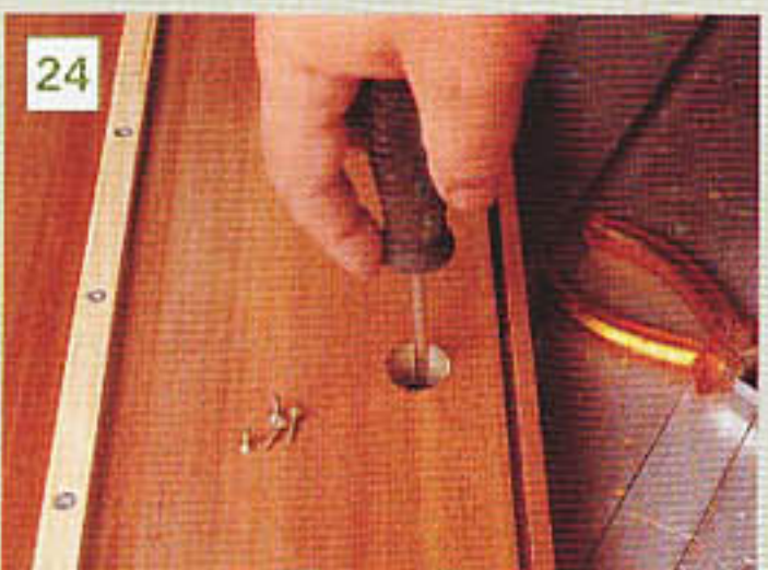
24 With the sliding baseboard inverted, the upper disc of MDF which forms the top rotating baseboard can be fitted using the access hole for driving the screws
